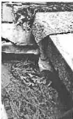
Clogged gutter leading to corrosion.
