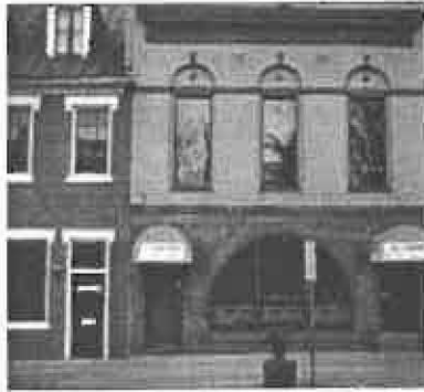
Incompatible replacement storefront and inappropriate window alteration.
