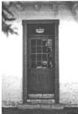
Operable over-the-door transom providing cross ventilation.
